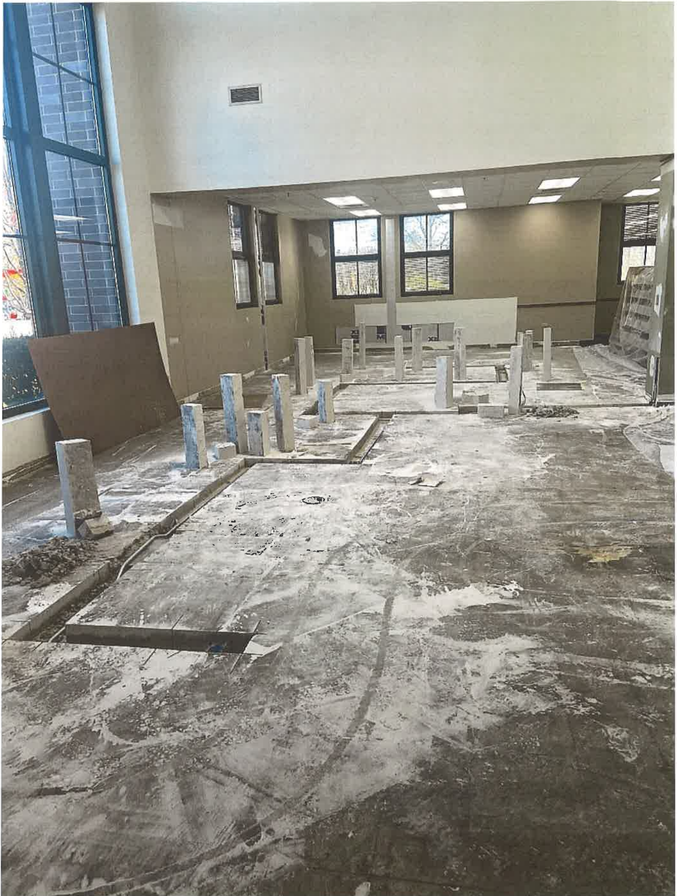
Looking west across new cafe space. They are trenching for electrical work
